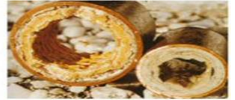
Lime scale has almost blocked these pipes
