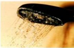
Blocked Shower head
