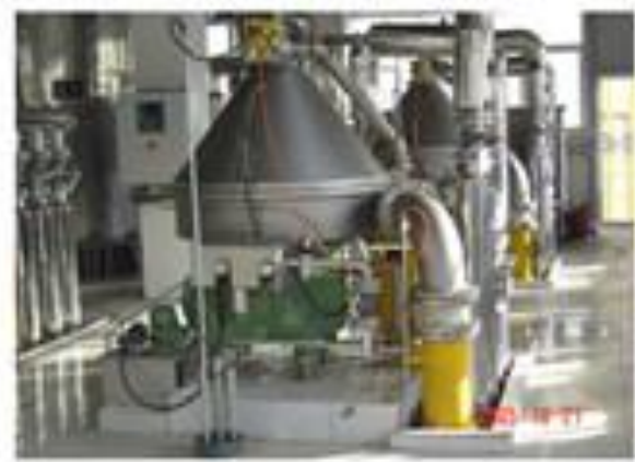
Third step Oil refinery
