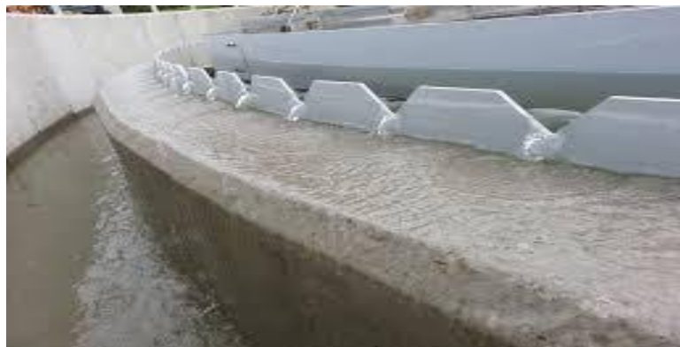
Fig.18 V-noches outlet weir
