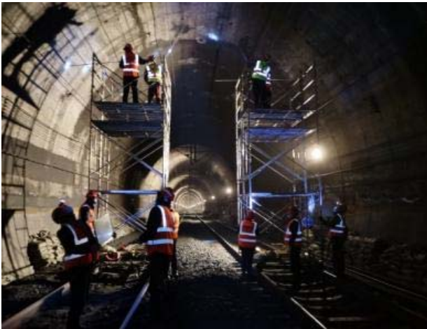
Fig. 12. Tunnel manual tapping detection
