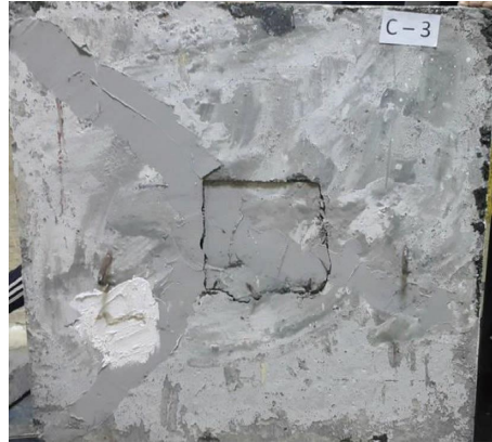
FIGURE 12: Punching shear failure.
