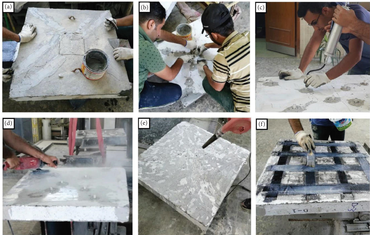
FIGURE 5: Repair process of control slabs after testing: (a) sealing the cracks on the compression side with Sikadur-31 material, (b) making holes and installing surface parkers on the tension side, (c) injecting Sikadur-52 LP material, (d) flattening the surface, (e) surface cleaning, and (f) applying the CFRP composite system.
