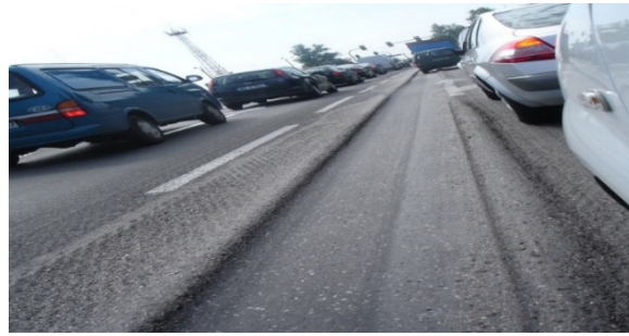
Fig. 1: Rutting in intersection approach.
