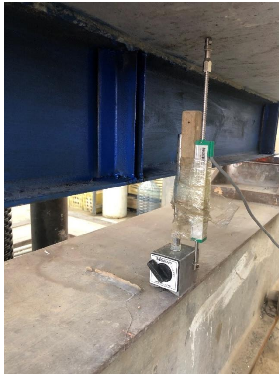
Fig.20 deflection gage sensor.
