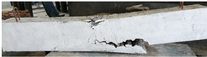
Fig. 8. SB1 Beam delamination.
