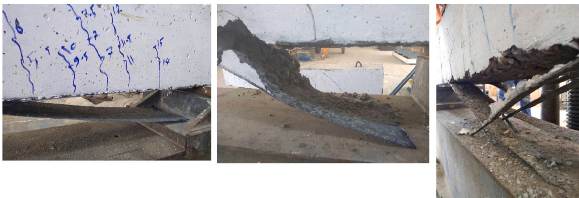
Fig. 12. Closer shoot for different mode of failure a) debonding b) cover delamination c) fiber rupture.
