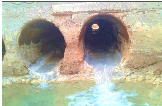
Figure7. The pipes under the paved road which pass the water from the drainage canal to Khor Al-Zubair waterway.
