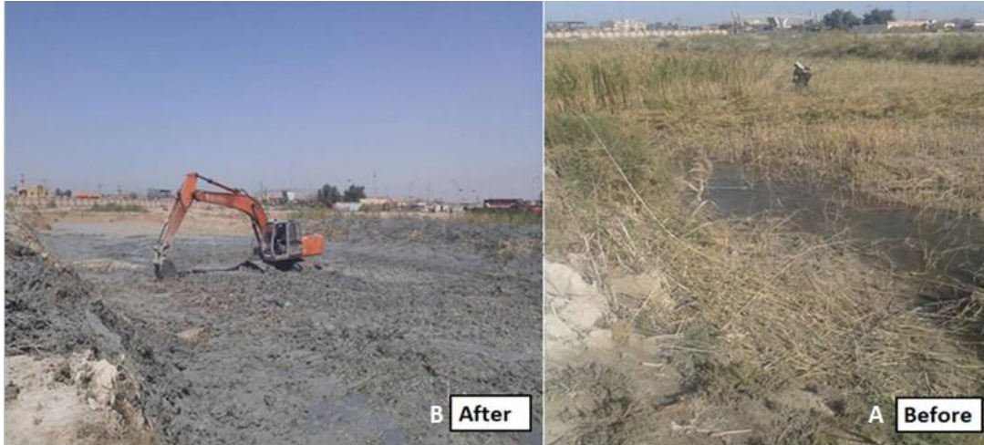
Pic. 1. Shrimp pond A = before, B = after remove all vegetation during the first stage.
