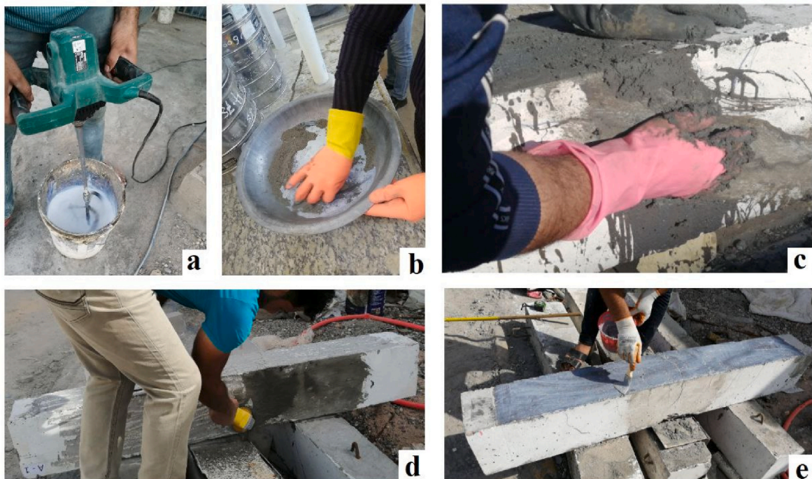
Fig. 5. Repair procedure a) blending the SikalateX with water b) mixing cement and sand with the wet part c) applying the repair mortar on the damaged area d) flatten and roughen the tension surface e) applying the epoxy resin then the fabric.
