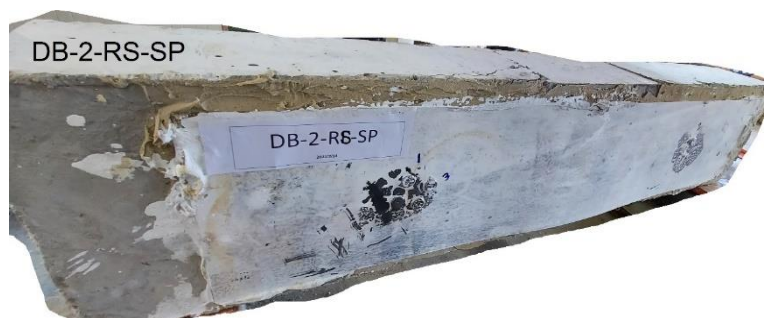
Figure (23): Failure mode for Rehabilitation Deep Beam with ( a/d=2 ) fail in shear - DB-2-RS-SP
