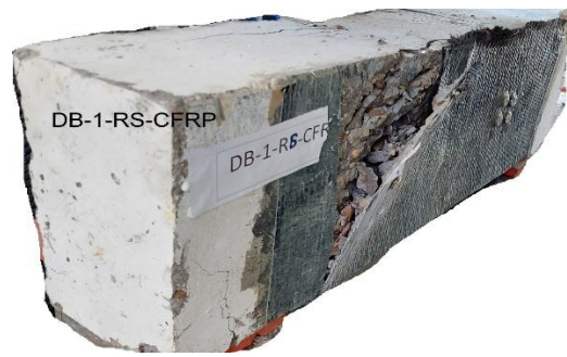
Figure (10): Failure mode for Rehabilitated Deep Beam with (a/d=1) failed in shear - DB-1-RS-CFRP
