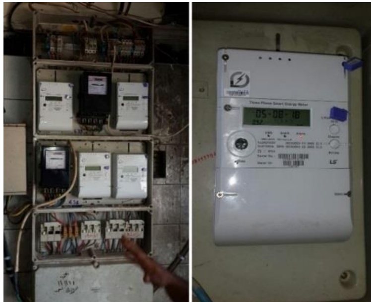
Figure 2. The smart meter installed in two sectors in Baghdad.
