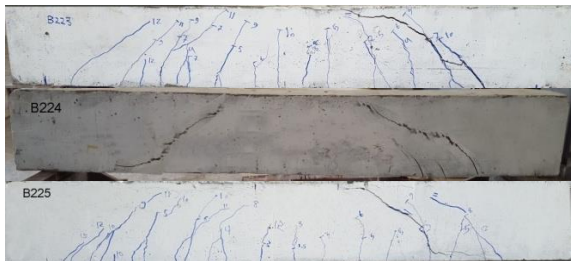
Figure 8: Crack pattern of group four ferrocement beams
