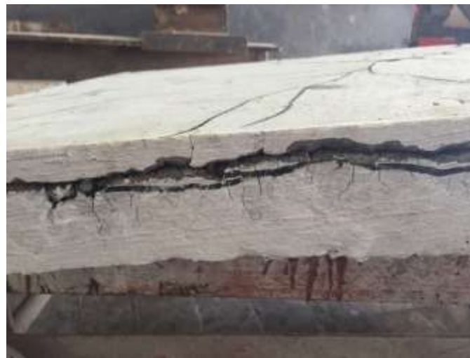
Fig.7: Debonding of ferrocement layer
