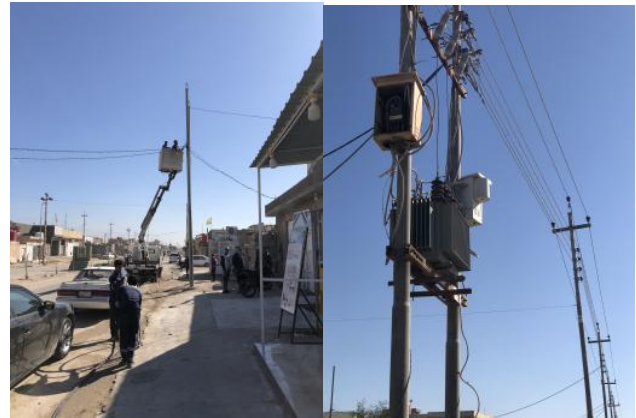
Poor Performance Transformers and a Part of the Maintenance Work in the City in 2021
