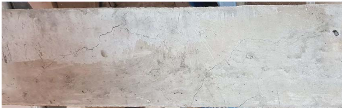
Figure 7. Crack pattern of fiber specimens.
