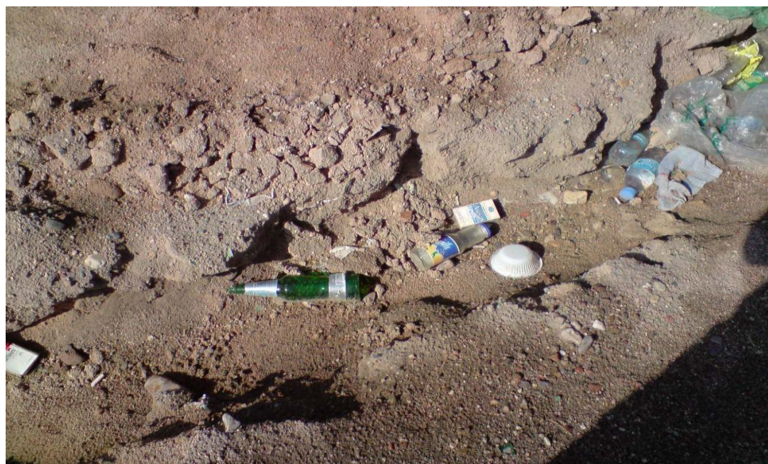
Fig.(3) Study embankment with remarked gully erosion
