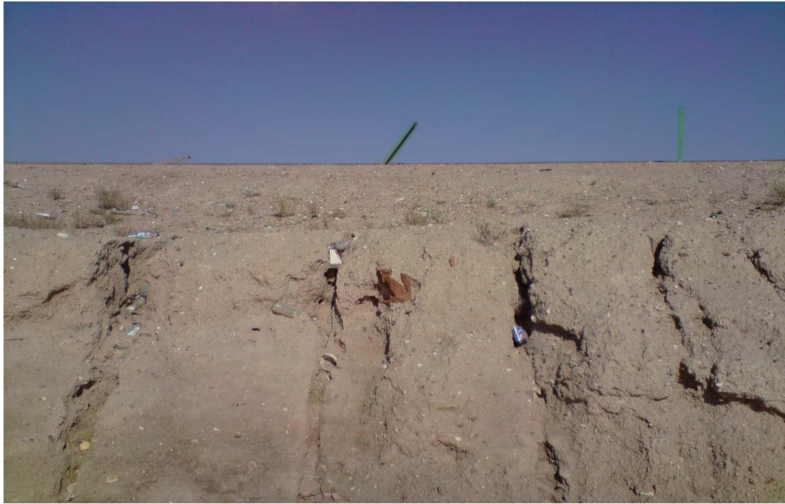
Fig.(4) Study embankment with remarked gully erosion
