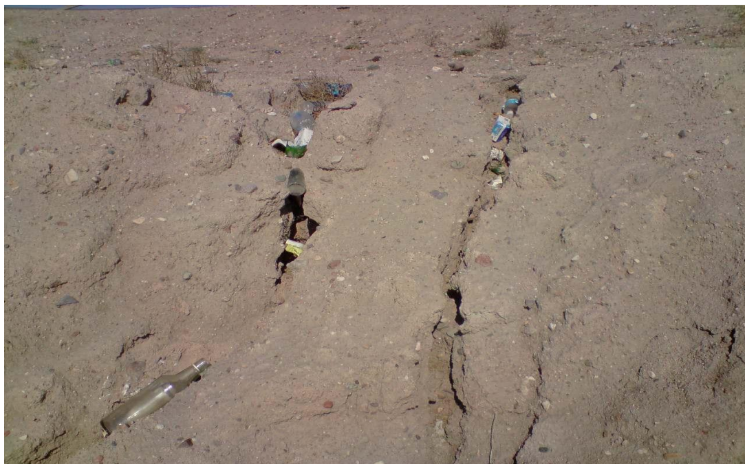
Fig.(2) Study embankment with remarked gully erosion
