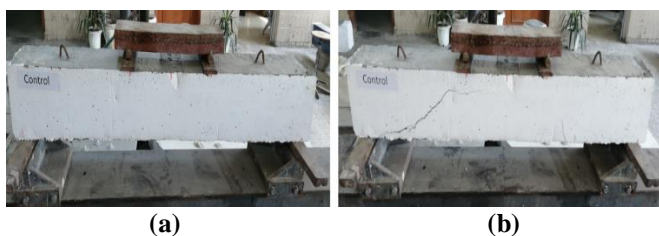
Fig. 10 The control beam (a) before the test and (b) after the failure.
