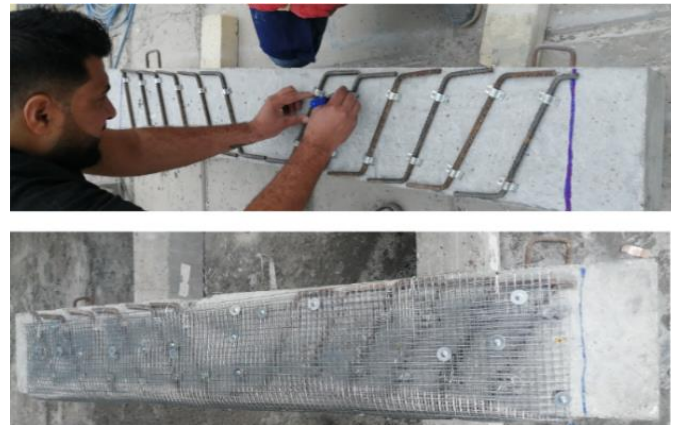
Fig. 7 The configuration of the externally bonded steel rebars used in the strengthening of the beam (S.-J. + Ferrocement + R).
