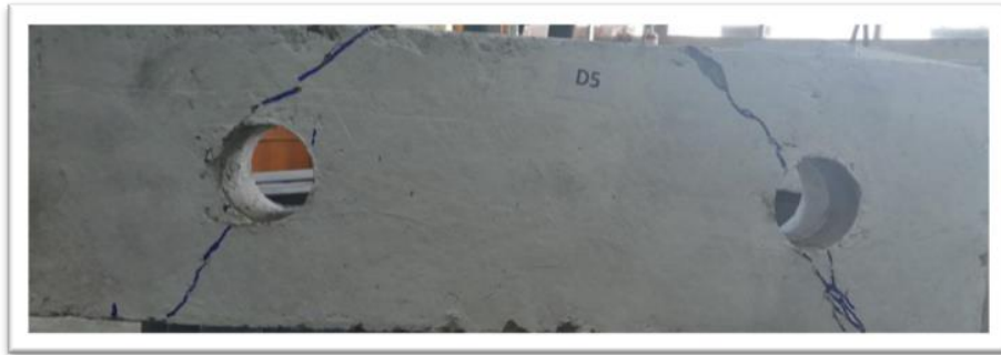
Figure 8. Shear cracks pattern of D5
