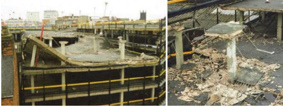
Figure (5): Upper floor collapse of Wolverhampton parking (UK) [10]
