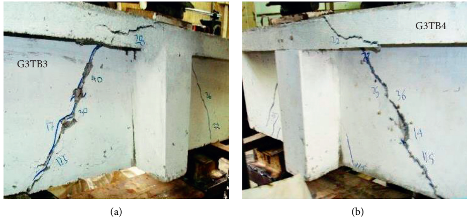
FIGURE 8: Crack pattern for indirectly loaded beams without shear reinforcement.
