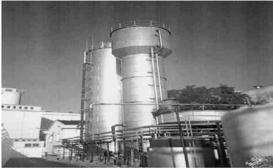
Fig. 13: Full scale Paques CIRCOX (front, 140 m 3 ) and IC (back, 385 m 3 ) reactors at a brewery in Brazil (Heijnen et al. , 1991)
