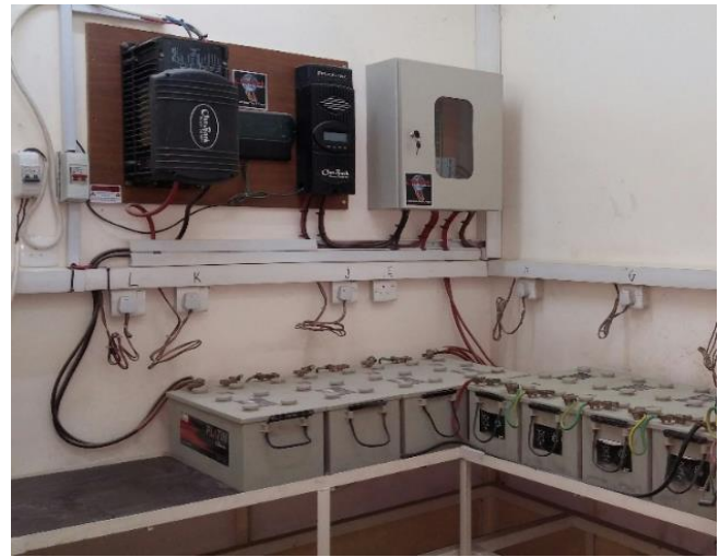
Fig. 2-b Stand Alone 3 KW PV system
