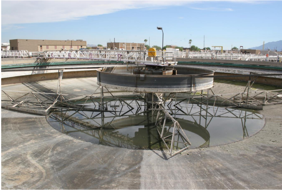
Fig.(4-6) Photo of primary sedimentation tank
