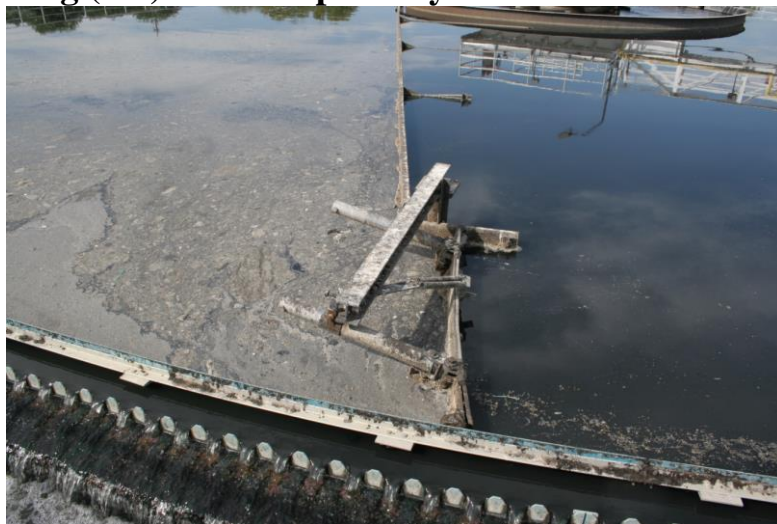
Fig.(4-7) Outlet weir, scum baffle and skimmer
